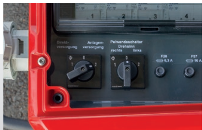
„Direct supply - system supply“ switch
